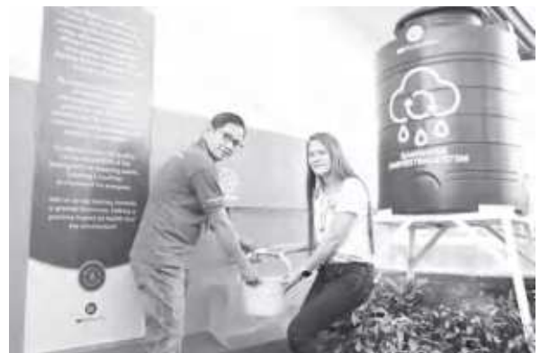
The rainwater catchment system helps lessen the center's reliance on municipal sources and contribute to water conservation efforts.
