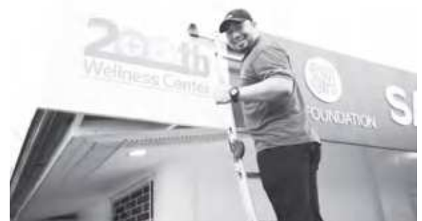
SM Foundation's Senior Project Manager Albert Uy places the 200th Wellness Center marker as they complete the final stages of the renovation.
